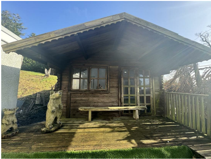
Summerhouse housing the hot tub. Free standing Worcester oil fired central heating boiler.
